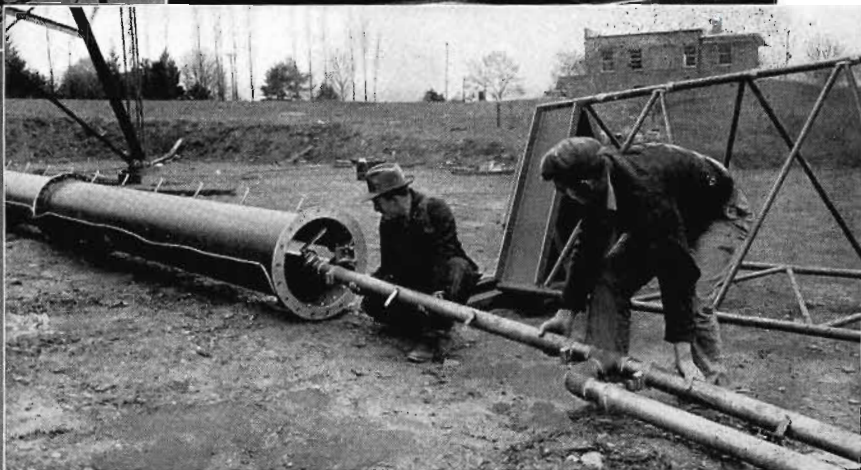
Inserting the transmission line harness into the two-section Pylon at WSBA-FM, York, Pa.
