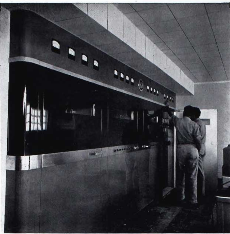
◀ At the power control section of the five kilowatt transmitter, Type BTA-5F, at KOOL, Phoenix, Ariz.
